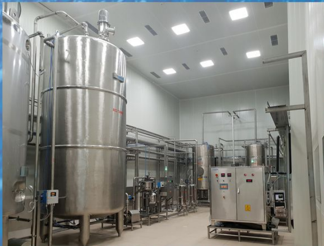
OZONE PLANT AT SITE
